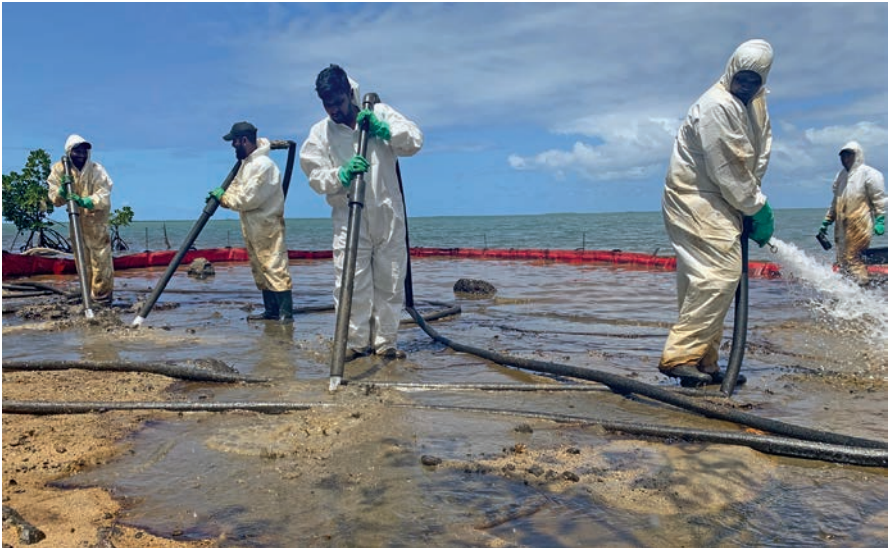
Flushing oil from substrate, Mauritius
